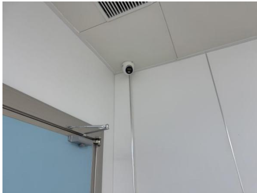
PET/CT 机房内摄像头
